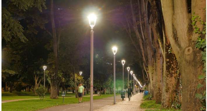
Streetlight Upgrade Program
